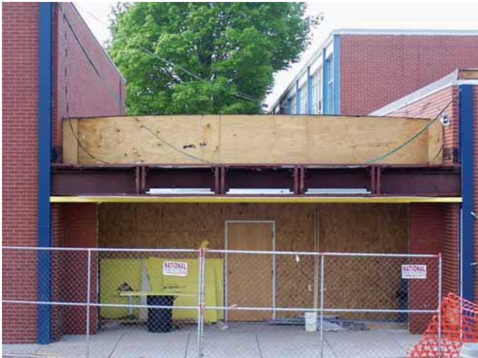
The construction of the new façade for the entrance to the Parish Center.
